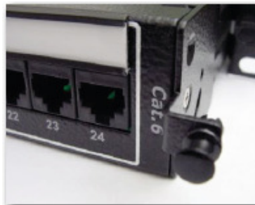
Data and Voice patch panels
